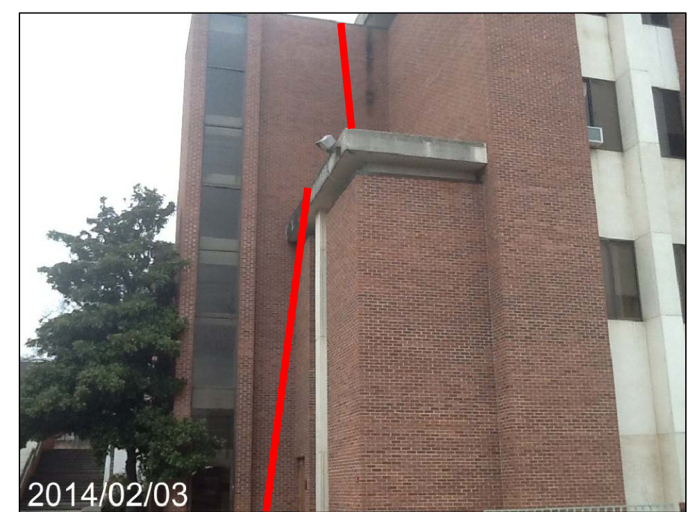
SOUTHWEST ELEVATION: • RED LINE DENOTES APPROVED ACCESS POINTS FOR SECTORS E AND F.
