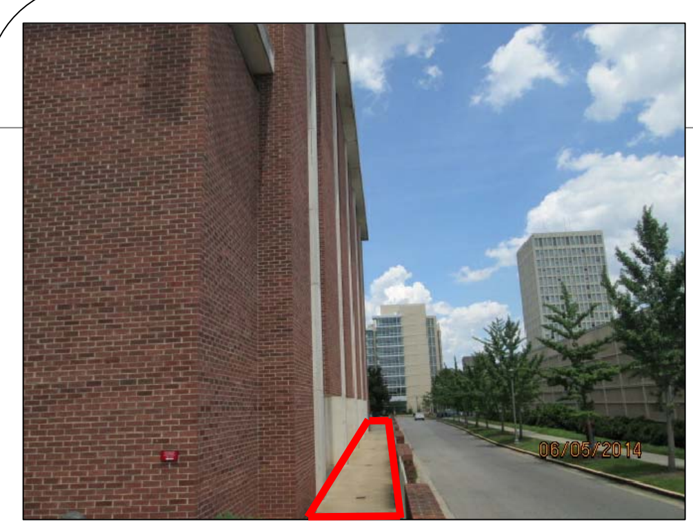
• WORK TO BE COMPLETED FROM SCAFFOLDING. RED LINE DENOTES APPROVED SCAFFOLDING STAGING AREA.
