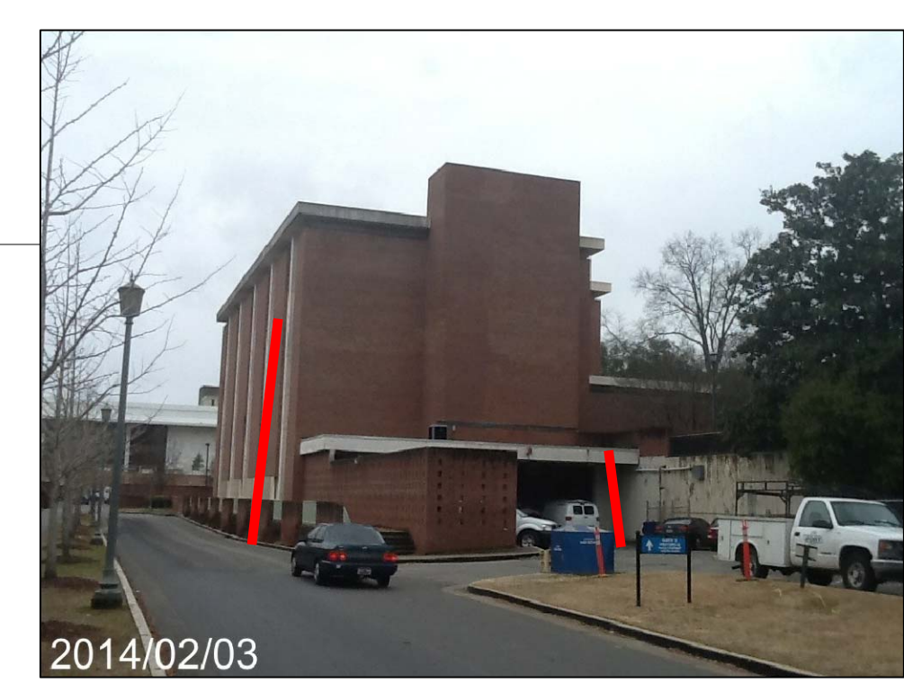
EAST ELEVATION: • WORK TO BE COMPLETED FROM SCAFFOLDING. RED LINE DENOTES APPROVED SCAFFOLDING STAGING AREA FOR SOUTHEAST ELEVATION AND ACCESS TO SECTOR D. LOADING DOCK AREA APPROVED FOR SMALL CRANE. PROVIDE MINIMUM 10 FOOT FIRE LANE IN LOCATION APPROVED BY OWNER AT LOADING DOCK.
